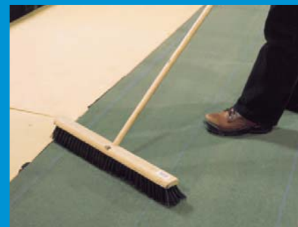
3 Broom or roll the base sheet to maximize adherence and eliminate voids.
