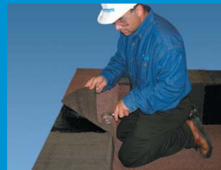
7 Install the cap sheet flashing membrane in a full bed of adhesive.
